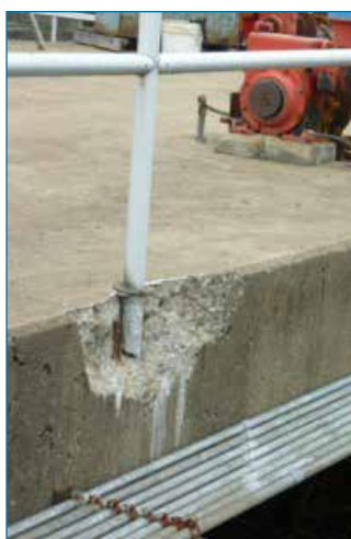
Deteriorated concrete at the final settling tanks.
