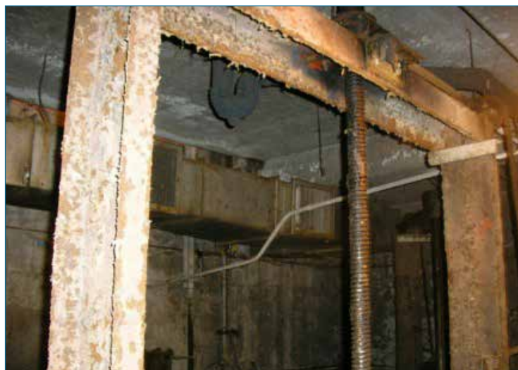
Corrosion at the raw waste pump station.
